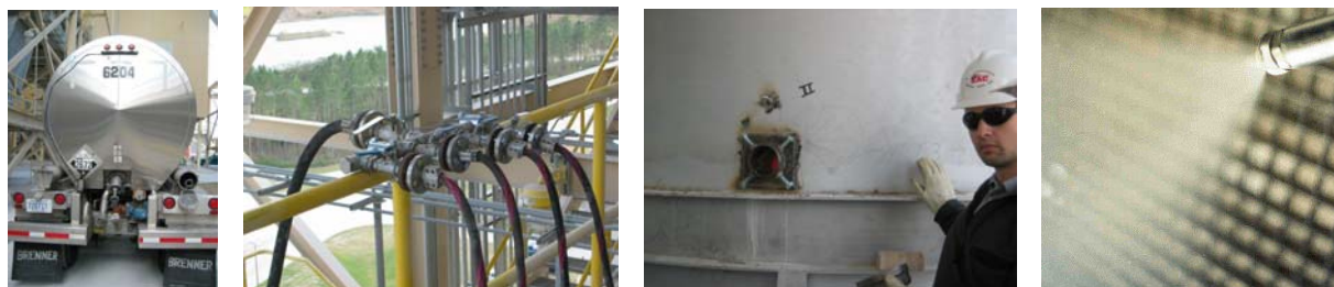
Figure 10. Aqueous Ammonia Supply Truck, Compressed Air, One of Four Ports, An Injector
