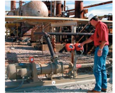
SP75 amine gas service application Big Lake, Texas
