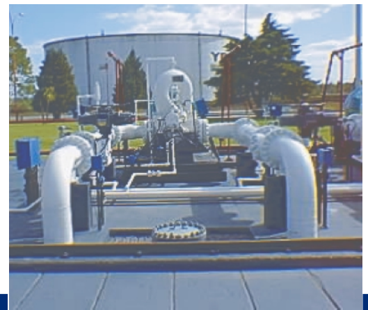
Figure 3 : Berisso Storage, Pump and Throttling Valve
