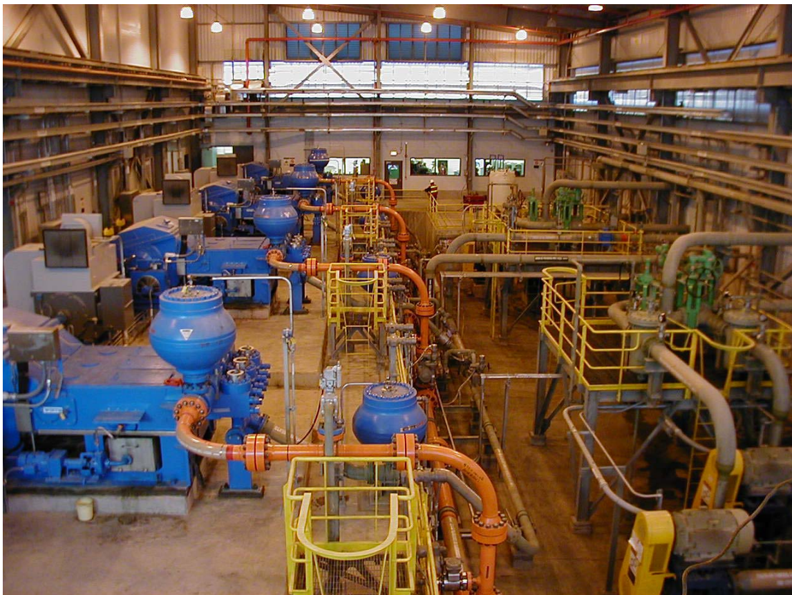
Figure 1: Pump Station PS1
