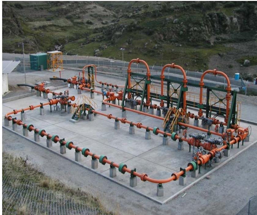
Figure 10: Choke station with vertical choke loops
