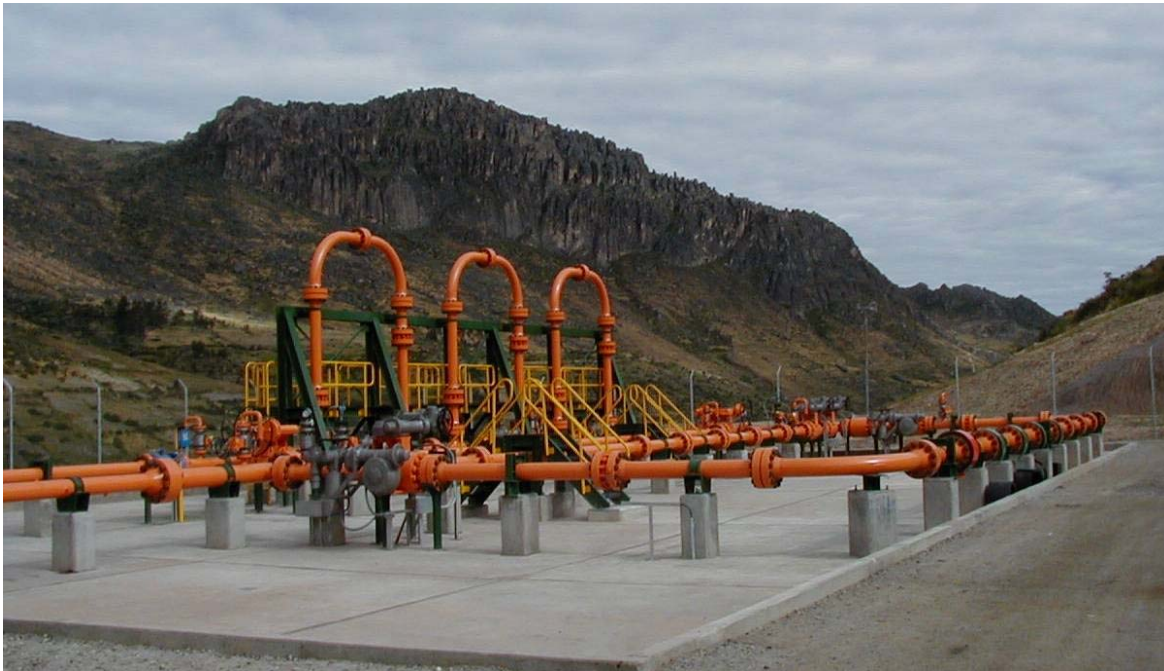
Figure 2: Valve Station 1/Choke Station
