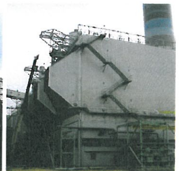
• Taean Thermal Power Plant Units 7~ 8
