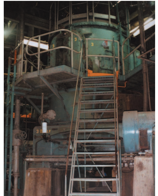
Combustion Engineering 783RP Bowl-Mill Coal Pulverizer.
