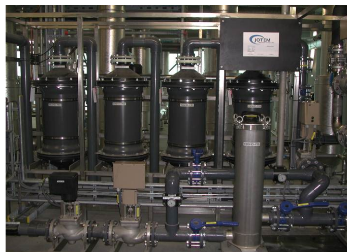
Figure 1: Oxygen removal system at Dutch power station
