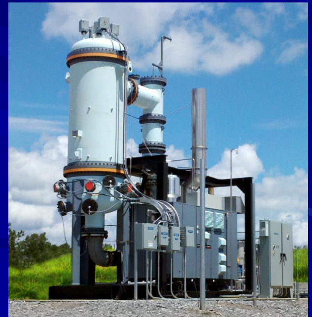
Flex Energy FP250 system
