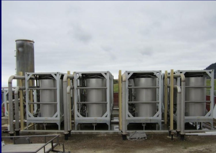
Gas Cleanup System
