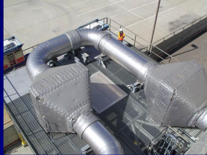
Oxidation Catalyst/SCR on elevated platform
