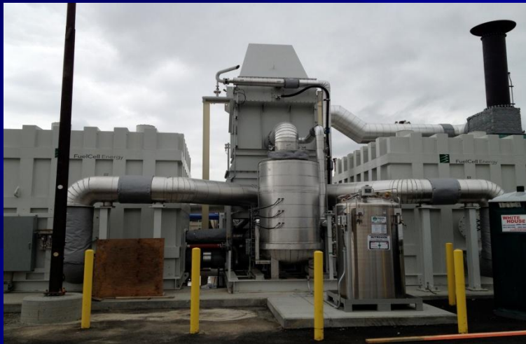
Fuel Cell Energy 2.8 MW unit
