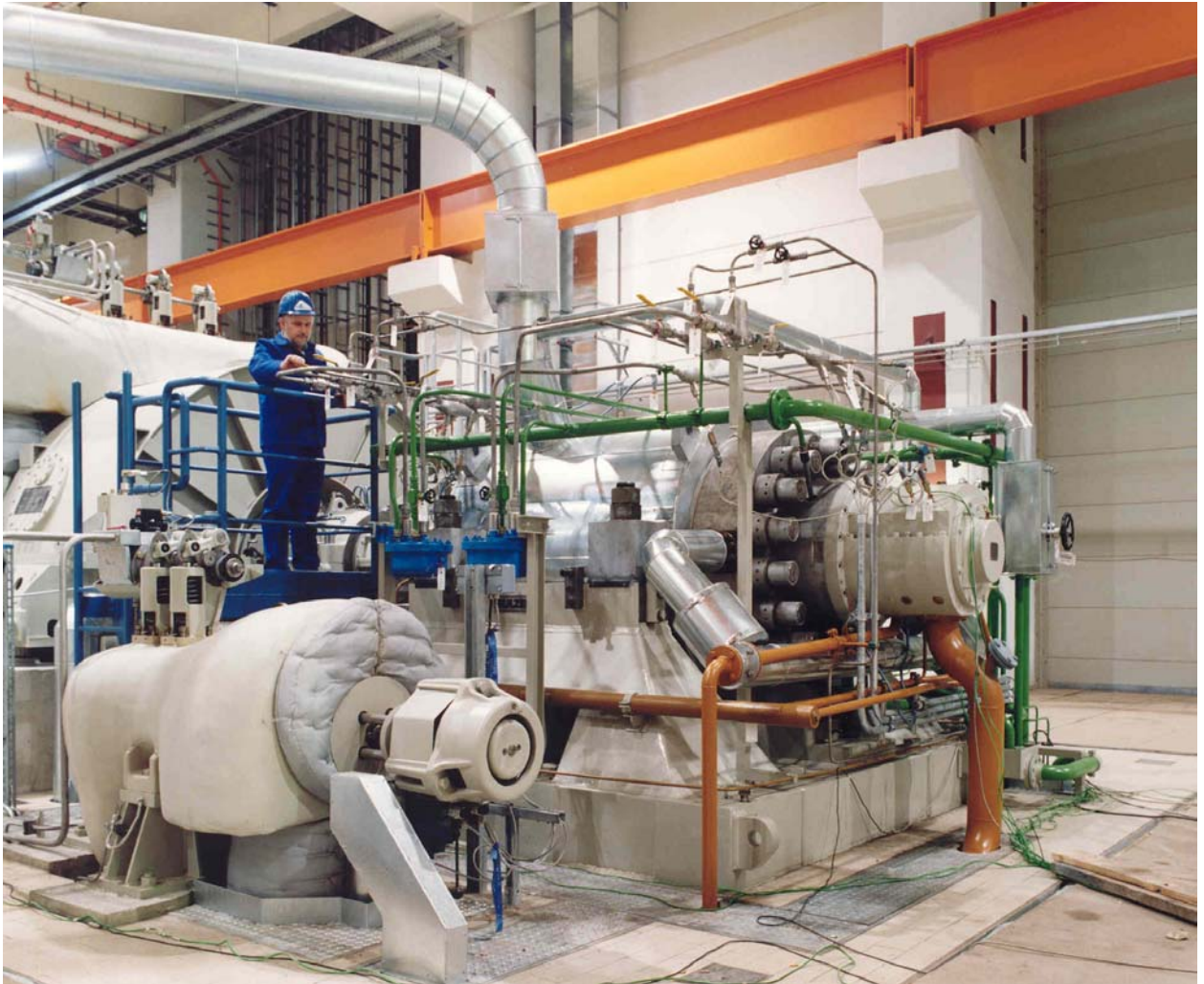
HPT type pump in the power station Lippendorf
