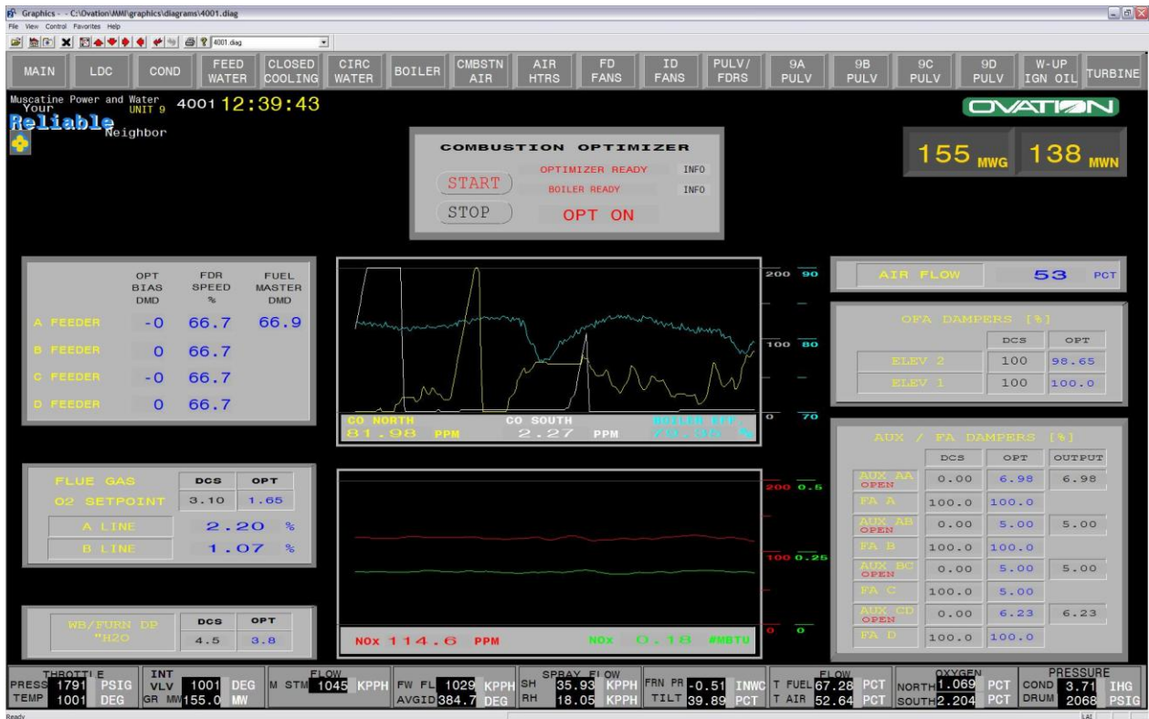
Figure # 12 Combustion Optimizer Control
