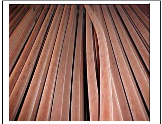
Figure 10 Buckled tube as a result of uneven condensate clearing
