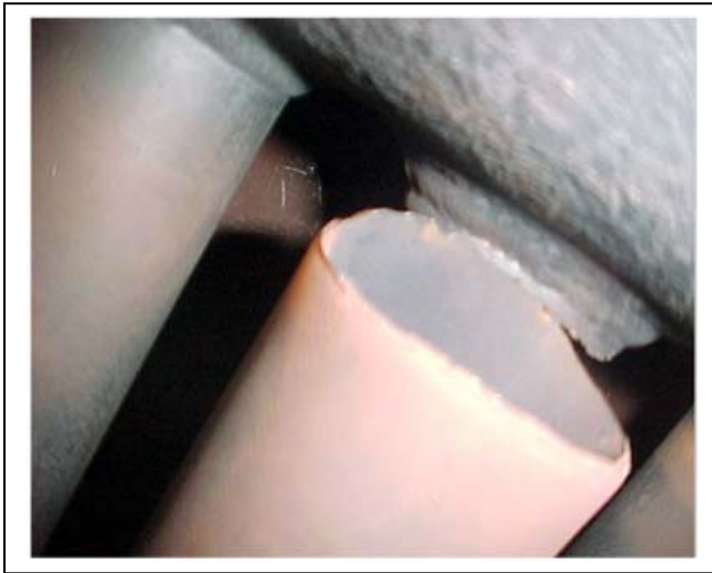
Figure 9 Damage caused by condensate quenching from desuperheater
