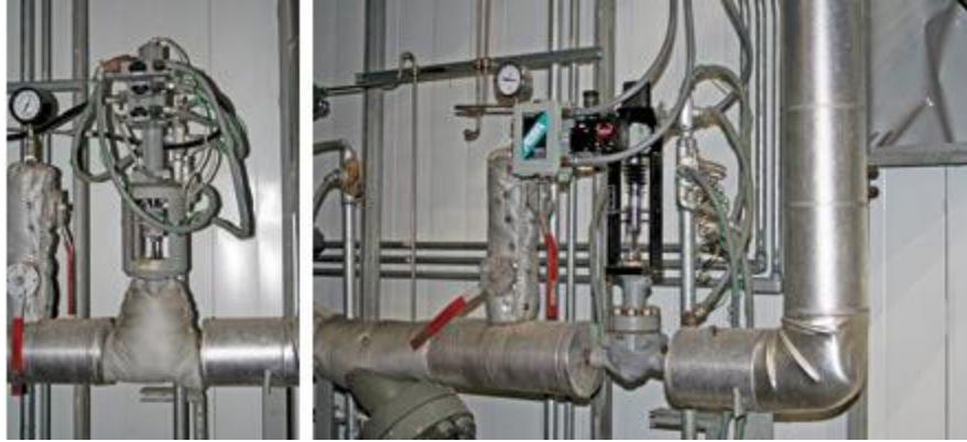
6. HP attemperator retrofit. Retrofit of a conventional hydraulic system actuator (left) to an Electraulic actuator (right) on the HP attemperator of a typical combined-cycle plant. Courtesy: Koso America Inc.
