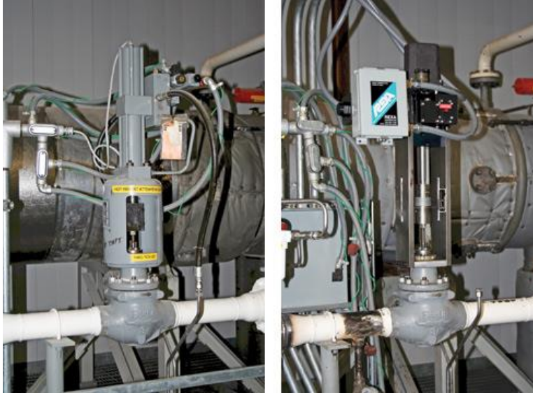
4. IP attemperator retrofit. Retrofit of a conventional hydraulic system actuator (top) to an Electrohydraulic actuator (bottom) on the IP attemperator of a typical combined-cycle plant. Courtesy: Koso America Inc.
