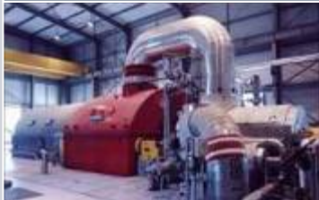
Steam Turbine Generators
