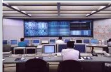
Instrumentation & Control Systems
