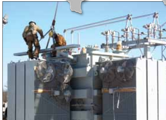
Top: Sunbelt locations across the US. Bottom: Sunbelt Transformer crew Field Dressing a 20 MVA Unit.
