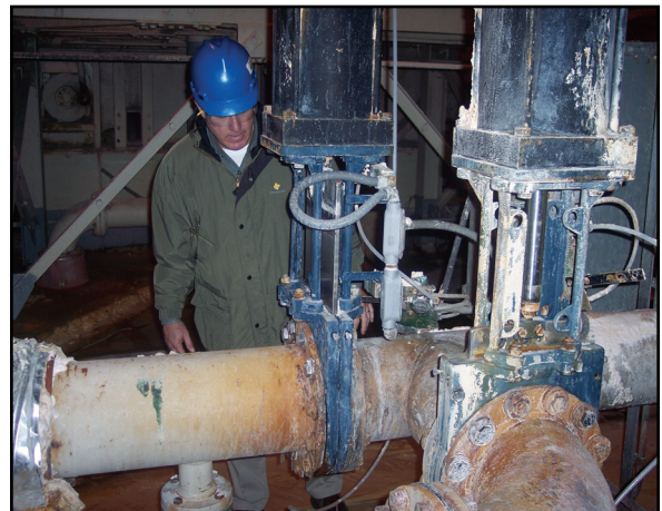
Seen here is a 10" actuated knife-gate valve (Model XS150ULV) from ITT on a gypsum slurry line for FGD service.
