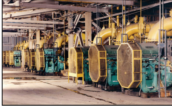
A bank of ITT rubber-lined slurry pumps on FGD service at a Missouri power plant.
