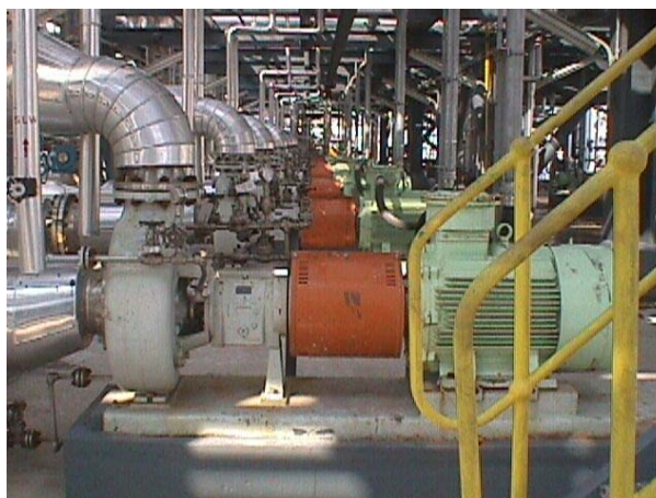
Seen here is the SECCO Acrylonitrile project with seven ITT Goulds brand 3196 pumps.
