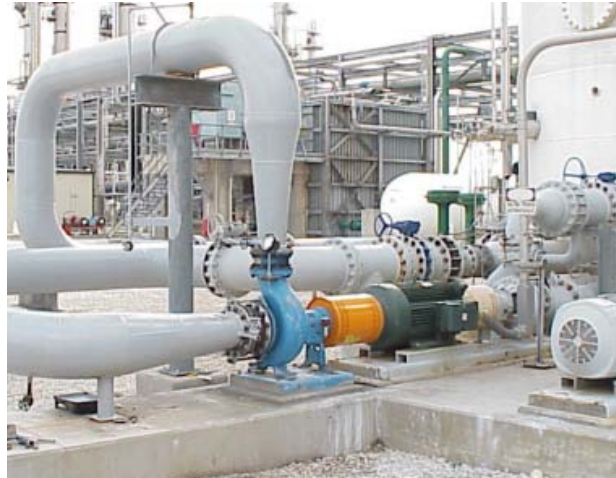
Seen here is the overall installation at Air Products including the 3196 chemical process pump from ITT's Goulds Pumps brand.
