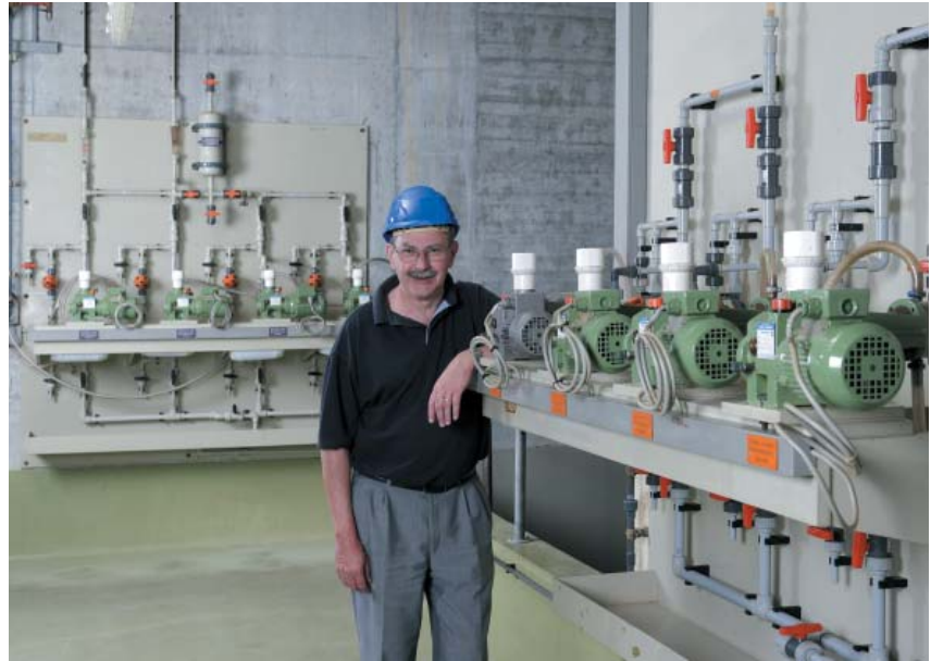
Bran+Luebbe pumps used for metering acid, caustic, heavy metal precipitant and flocculant solutions.
