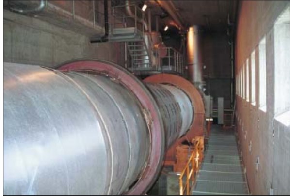
Rotary oven for drying and incinerating sludge
