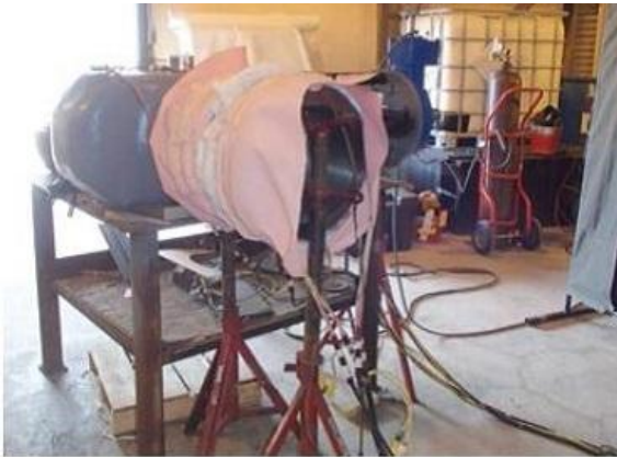
3. A 16 × 12 in. reducer was welded to the valve inlet to transition from the 16-in. line coming from the HRSG to the 12 in. stop valve. Heat-treatment step is in photo; all materials were P91. Welding and heat treatment were done at ground level
