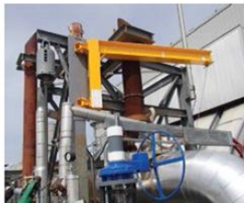
9. Jib crane was mounted to existing support steel and chained sideways for storage when not in use
