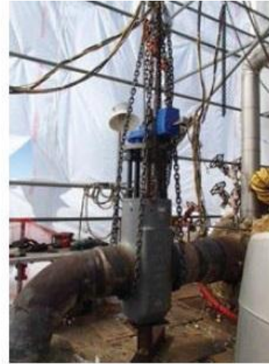
11. Several chainfalls were used to properly support and position the valve for welding
