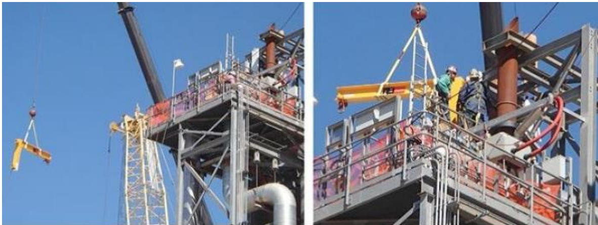
6, 7. Jib crane is "flown" to the top of the HRSG (left) and rigged in (right) to support the original valve during its removal
