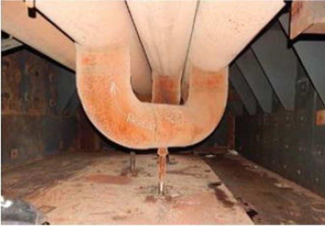
2. It's easy to understand why small drain pipes are affected by the behavior of superheater and reheater tubes
