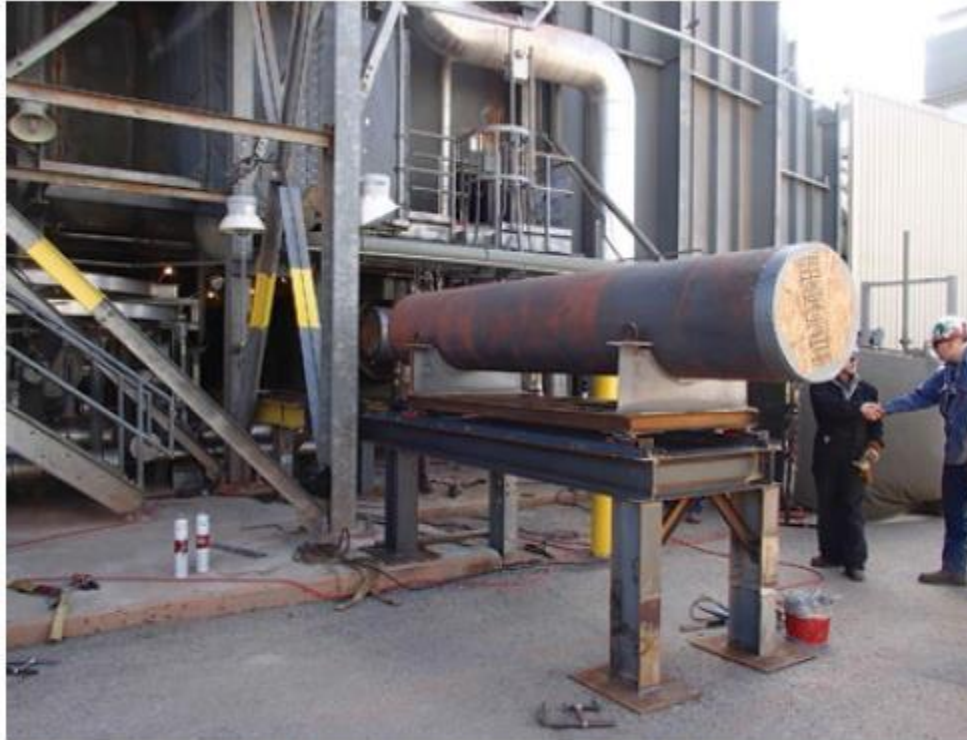
1. Replacing desuperheaters and associated piping is both time-consuming and expensive
