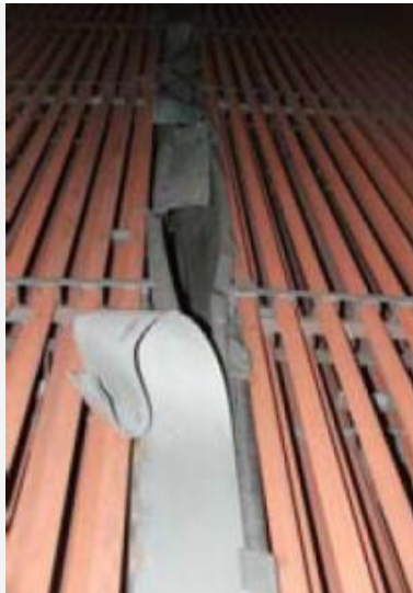
1. Failed baffle was designed to prevent turbine exhaust gas from bypassing heat-transfer surface by flowing between adjacent panels
