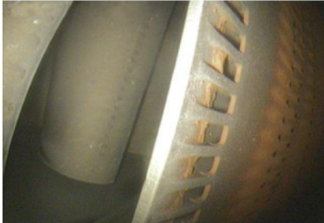
2. Fouling at the trailing edge of a first-stage nozzle. Engine was not equipped with HEPA filters
