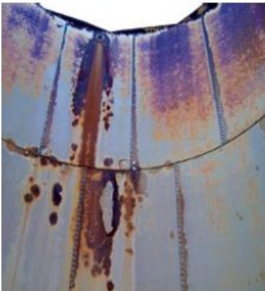
Internal shell of backwash tank
