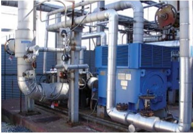
Boiler feed pump equipped with new motor driver
