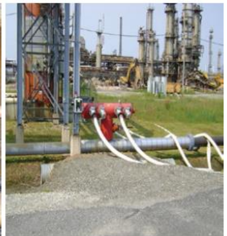
Firewater system supplied water to the plant
