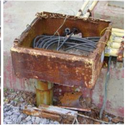
Junction box in poor condition
