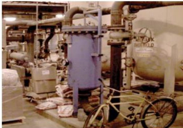
Water treatment and chemical room when plant was sold
