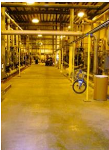
Water treatment area like new
