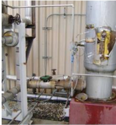
Do not stand on insulated pipes
