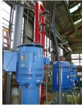
Service water and many other pumps reconditioned
