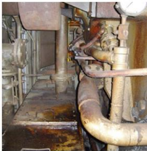
Gas turbine area suffered from lack of attention
