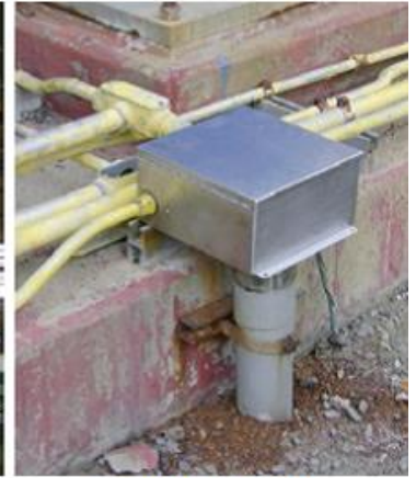
New junction box
