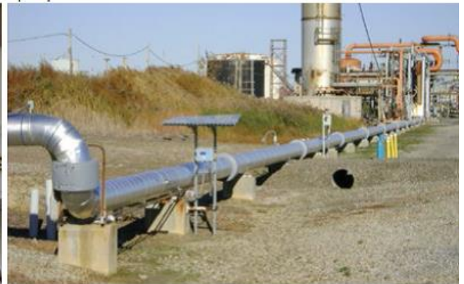
New raw-water line
