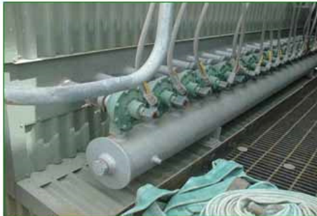
Figure 1 One of 8 manifolds fitted with 21 Goyen CA50T diaphragm valves.
