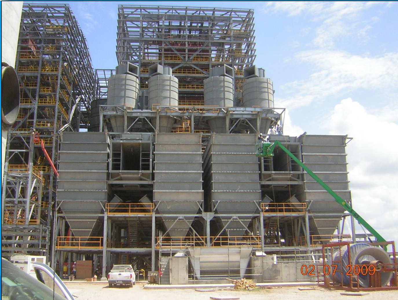
Dry Scrubber, Baghouse
