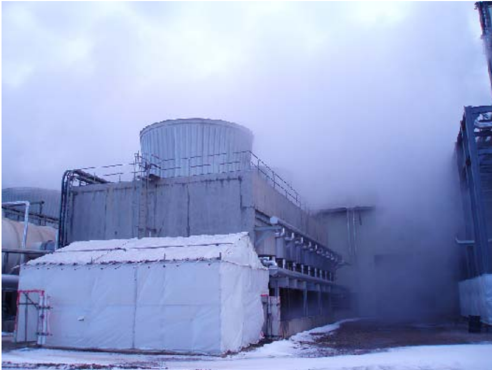
Figure 3-34. Aerosols Drifting from Cooling Tower to Gas Turbine Inlet (Courtesy of Camfil Farr)
