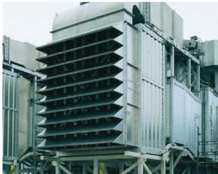
Figure 3-8. Weather Hood on Inlet Filtration System (Courtesy of Camfil Farr)
