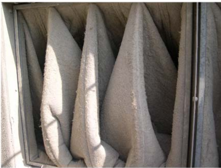
Bag filter loaded with limestone dust
