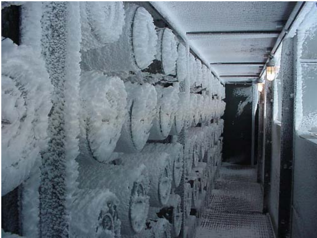
Figure 3-9. Cartridge Filters with Frost Build-Up Due to Cooling Tower Drift (Courtesy of Camfil Farr)
