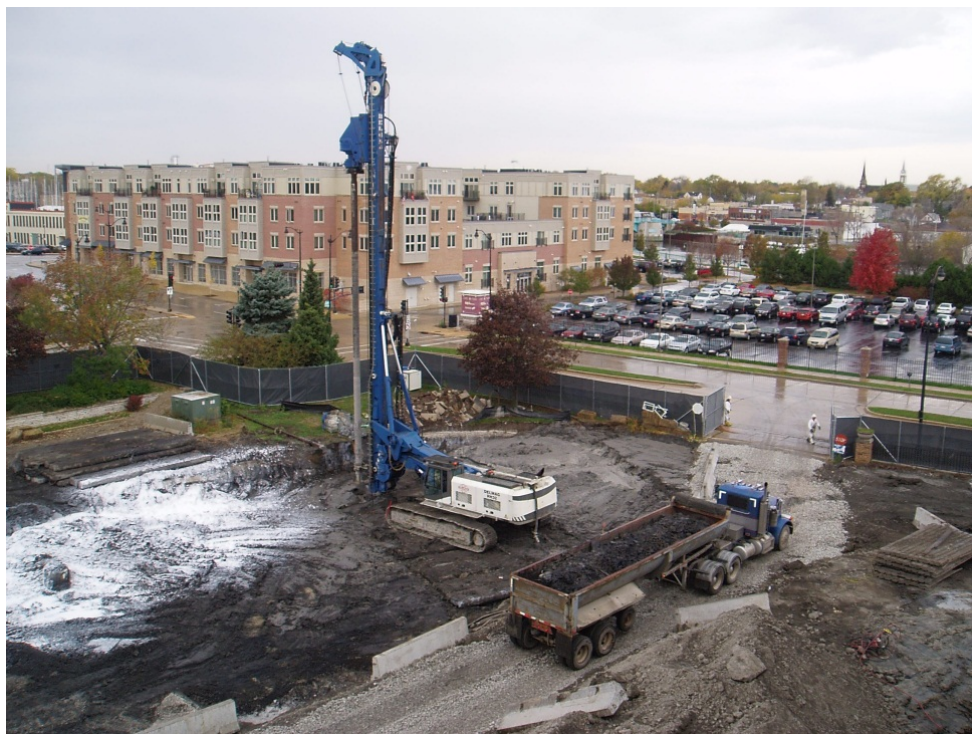
Figure 3 – Large Diameter Auger Mixing Using a Hydraulic Drilling Rig with Telescoping Boom
