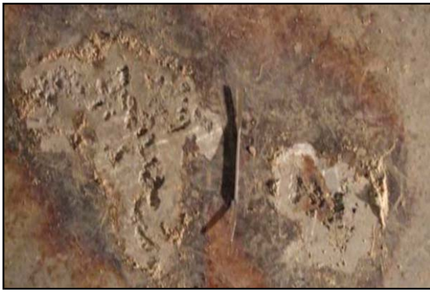
Fig. 12 Visible localized under-deposit corrosion.
