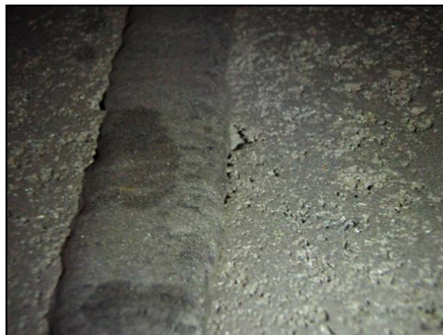
Fig. 1 Aggressive corrosion near vertical weld.
