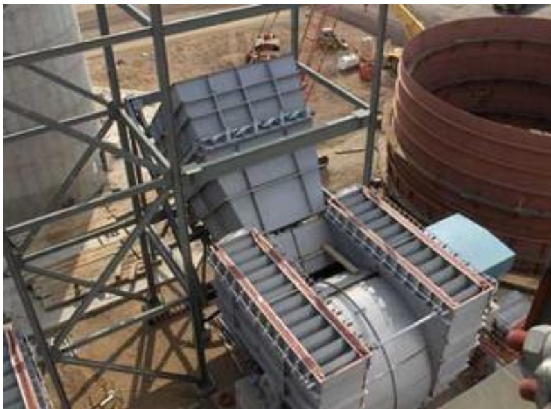
Induced draft fans being erected at the south unit of Weston 4. Photo courtesy Wisconsin Public Service.
