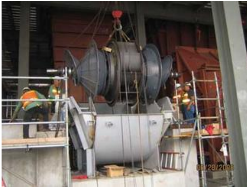
Primary air fan at Weston 4. Photo courtesy WPS.
