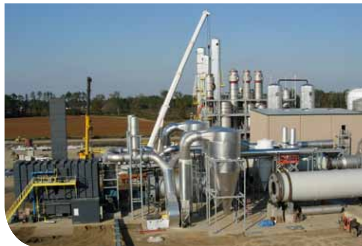
Integrated RTO with DDGS Dryers, Cooler, Cyclones and Ductwork
