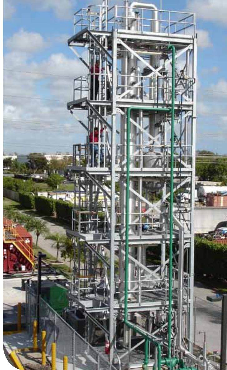
Wastewater Treatment from Pharmaceutical Plant
