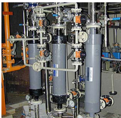
Liqui-Cel® Contactors efficiently treat ammonia wastewater in European facility
