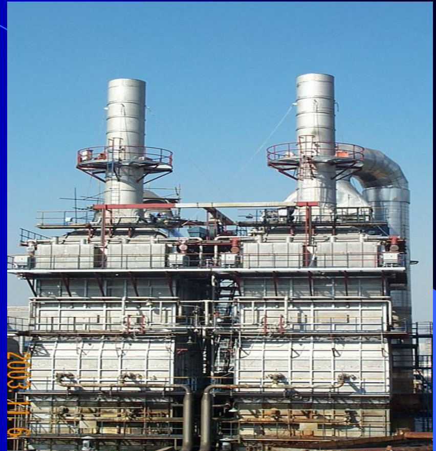
Beltran WESP: Heavy oil fired power station in petrochemical plant
