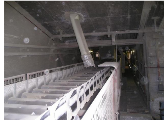
Bleedstream Injection on Clinker Apron Conveyor
