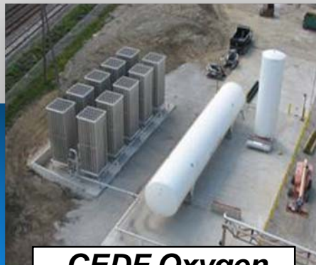
CEDF Oxygen Supply System
