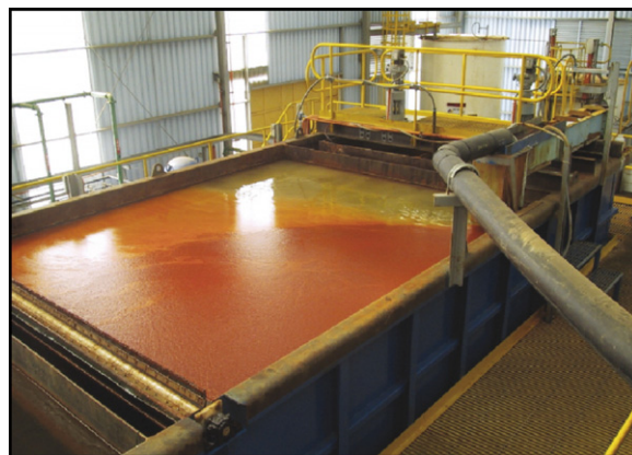
Fig. 8. Dissolved air flotation unit treating sulfides concentrates filtration water. The iron hydroxide is the adsorbing carrier for most of the ions (heavy metals and anions, sulfides and molybdates) in Chile (Rubio et al., 2002a,b).
