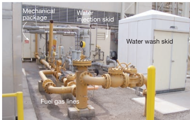
4-5. Demolishing everything in the photo, save the water wash skid, was first step
