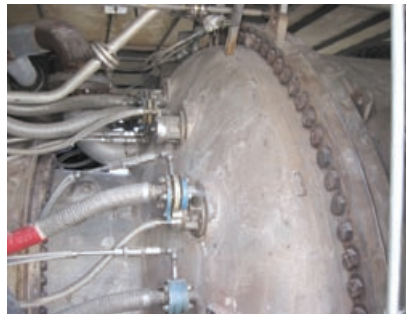
4-8. Insulation removed from OEM's CC case revealed end cover with gas line (large pipe) and other hardware
