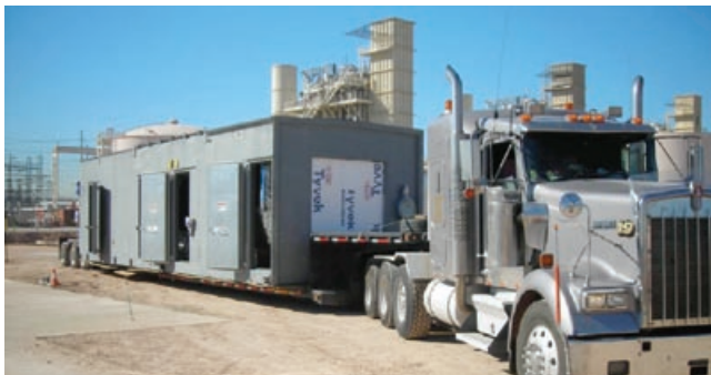
4-43. SwiftPacs are delivered in modules ready for installation. Here a gas-turbine package is brought to its pad
