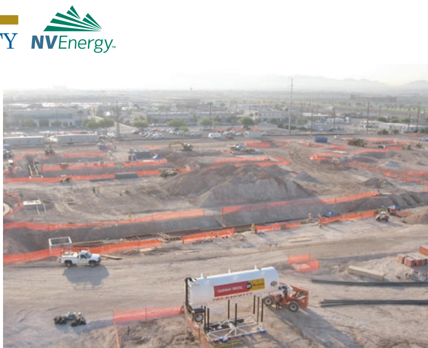
4-41. Site preparation for the 12 SwiftPacs in the early stages shows trenches to house the underground electrical distribution system and piping networks
