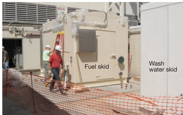
4-6. Wash water skid in Fig 5 retained its original foundation; PSM provided the new fuel skid
