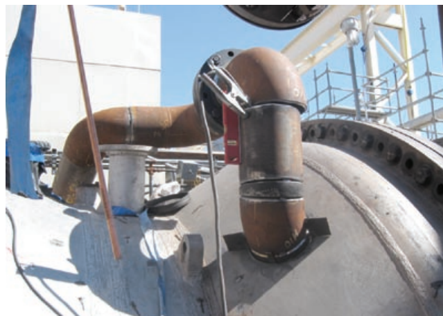
4-37. Compressor shell air is extracted to heat incoming ambient air
