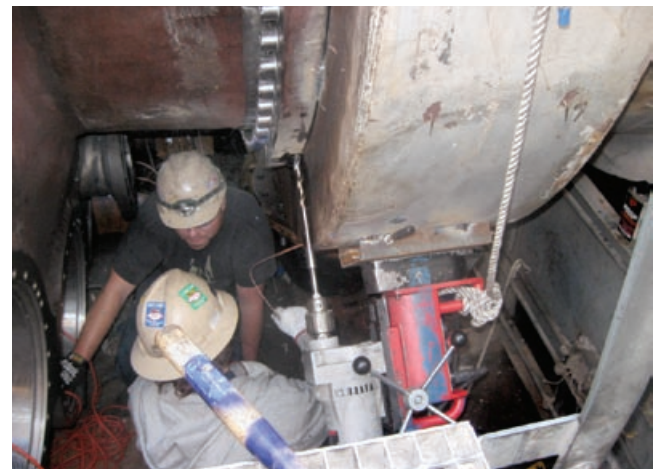
4-22. Alignment true, lower casing halves are drilled and doweled to hold their position
