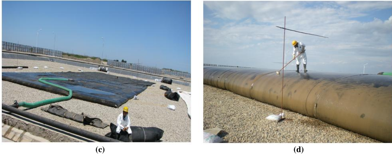
Figure 20. Full scale prototype geotextile tube trial performed at Tianjin Eco-City (a) lined drainage platform (b) unrolling of geotextile tube over drainage platform (c) filling geotextile tube with slurry (d) brushing of geotextile tube surface.
