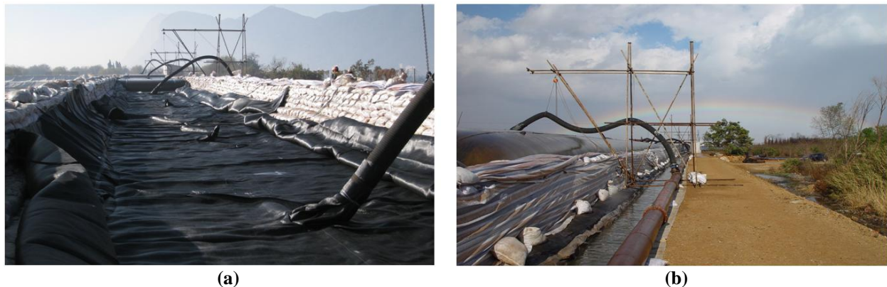
Figure 14. Geotextile tube dike at Liuyuan (a) geotextile tube ready for filling (b) filled geotextile tube.
