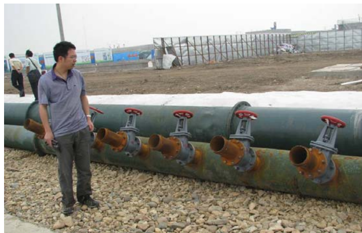
Figure 22. Incoming slurry delivery pipeline and multiple valve control.
