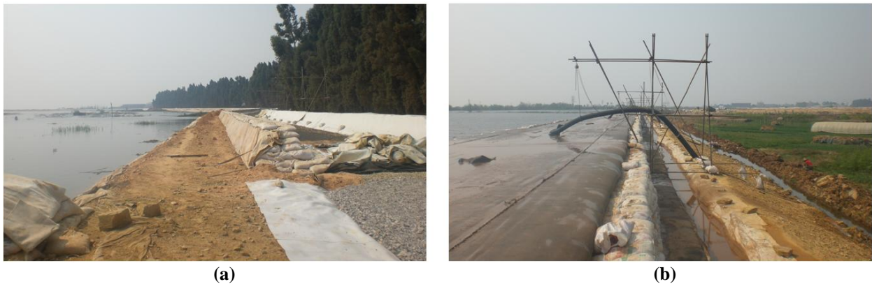
Figure 13. Geotextile tube dike at Fubaotang (a) subbase and sandbags (b) filling geotextile tube with slurry.
