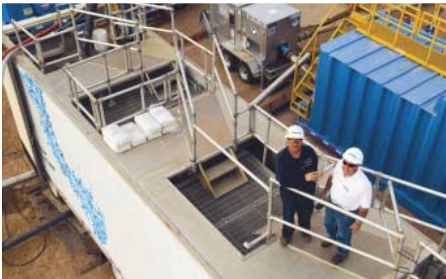
Siemens mobile purification system in Florida
