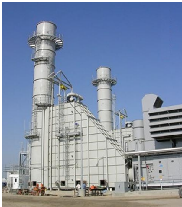
2. Typical simple cycle SCR. The SCR used on a simple cycle combustion turbine (CT) is located in an enclosure attached to the CT exhaust. Courtesy: Cormetech Inc.
