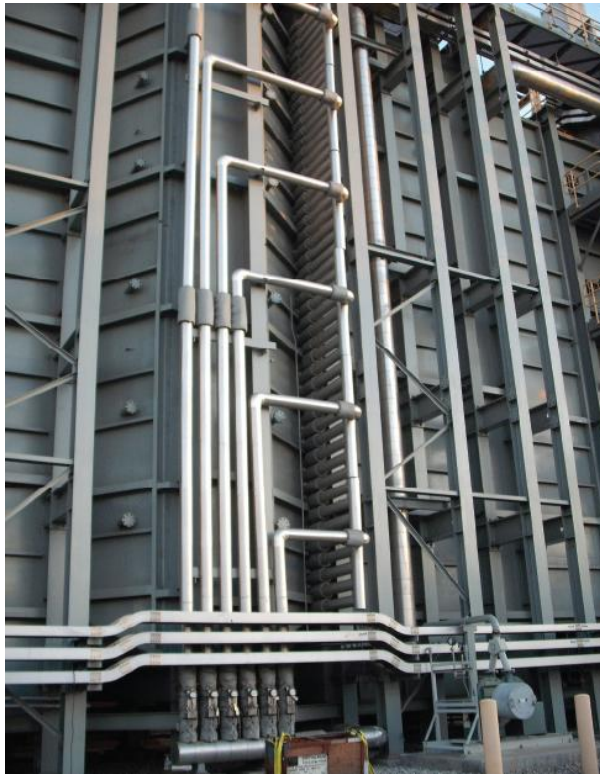
3. Typical HRSG ammonia injection grid. Ammonia reacts with the NO x in the exhaust gas stream over a catalyst to form molecular nitrogen and water vapor. If too much ammonia is used, unreacted ammonia may also leave the stack (ammonia slip). Courtesy: Cormetech Inc.
