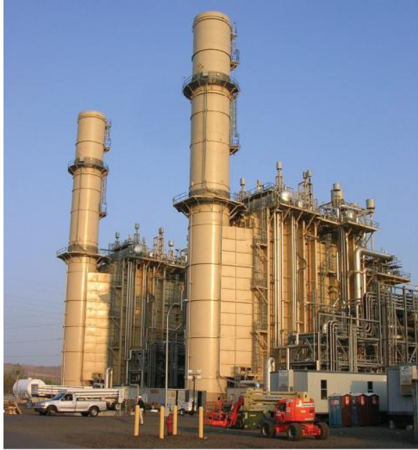
1. Typical combined cycle SCR. The SCR is a separate section located within the HRSG assembly where gas temperatures are optimal for SCR performance, typically 600F to 800F. Courtesy: Cormetech Inc.
