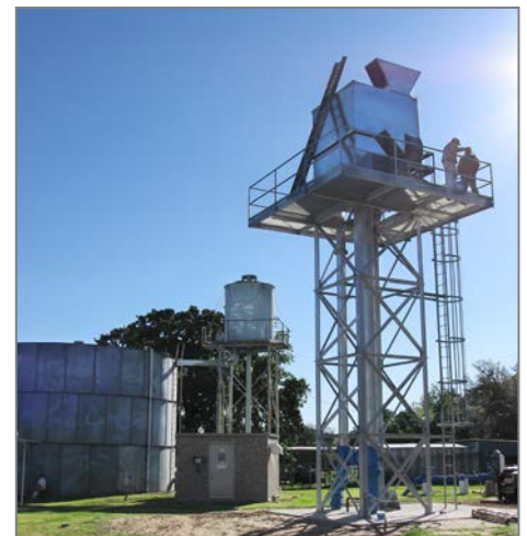
Existing and New Forced Draft Aerators
