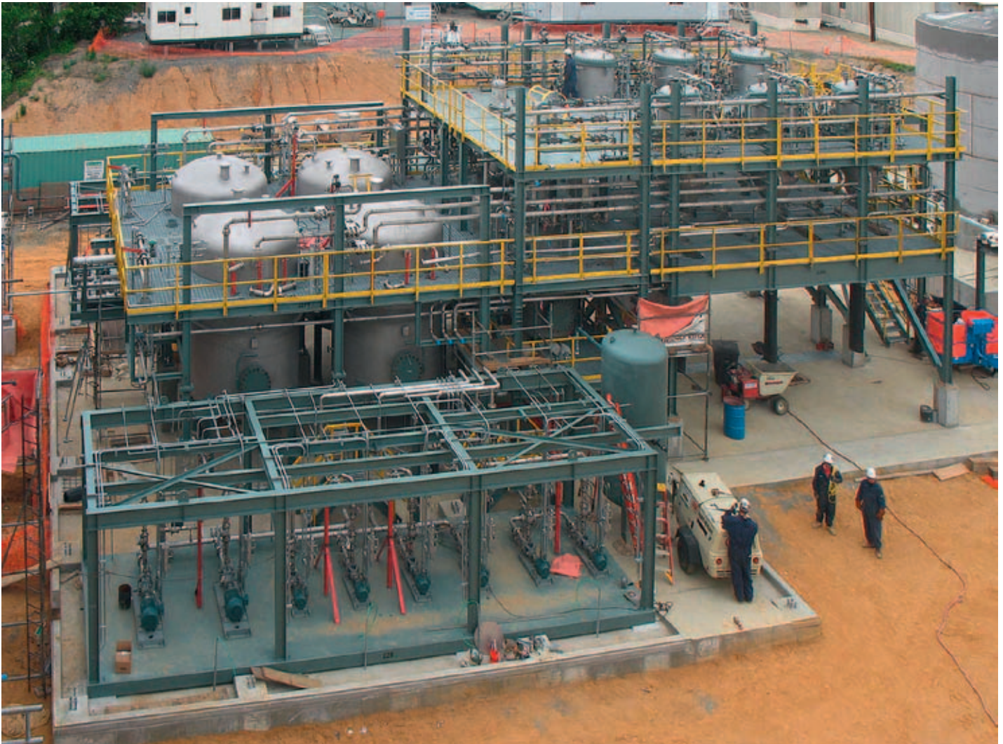
Duplex BHS candle filter system in a refinery with precoat tank and pumps, piping, wiring and complete PLC controls system which communication back to the refinery DCS. All filters, tanks and piping are heat traced and insulated.
