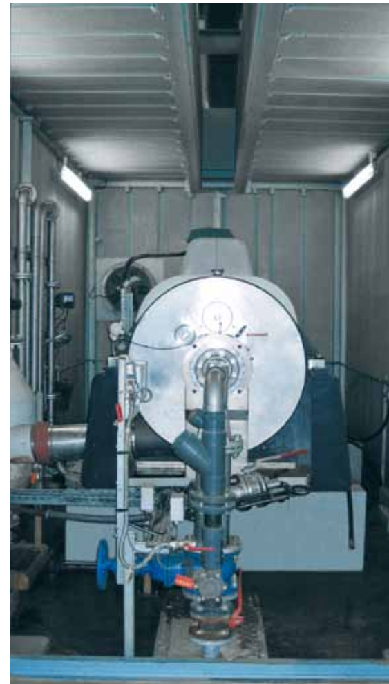
▲ Thickening-centrifuges, D7 series, installed for nitrification process
