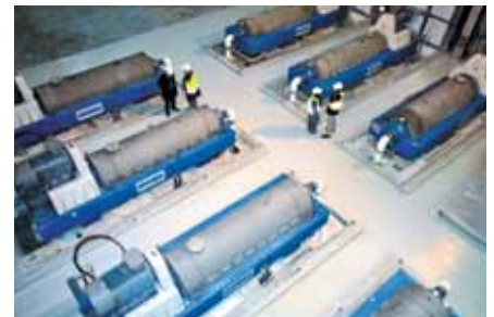
▲ Seven ANDRITZ D7series decanters at Tereos plant, France
