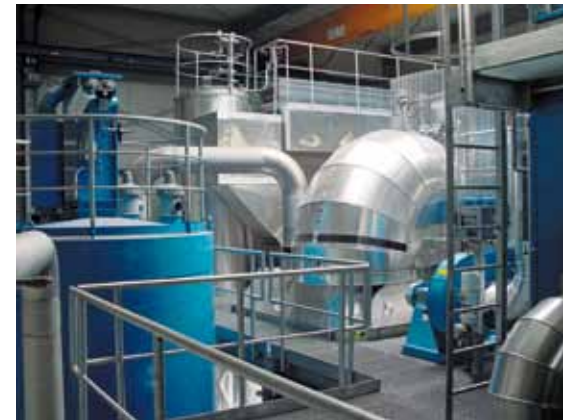
▲ EcoDry plant in Eferding, Austria
