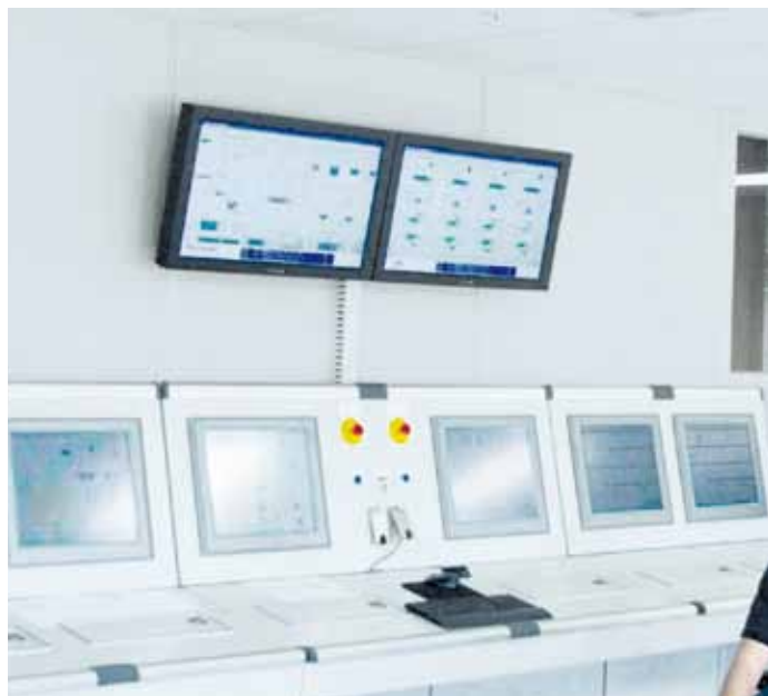
◀ Central control room of the dewatering plant, with 8 ANDRITZ membrane chamber filter presses
