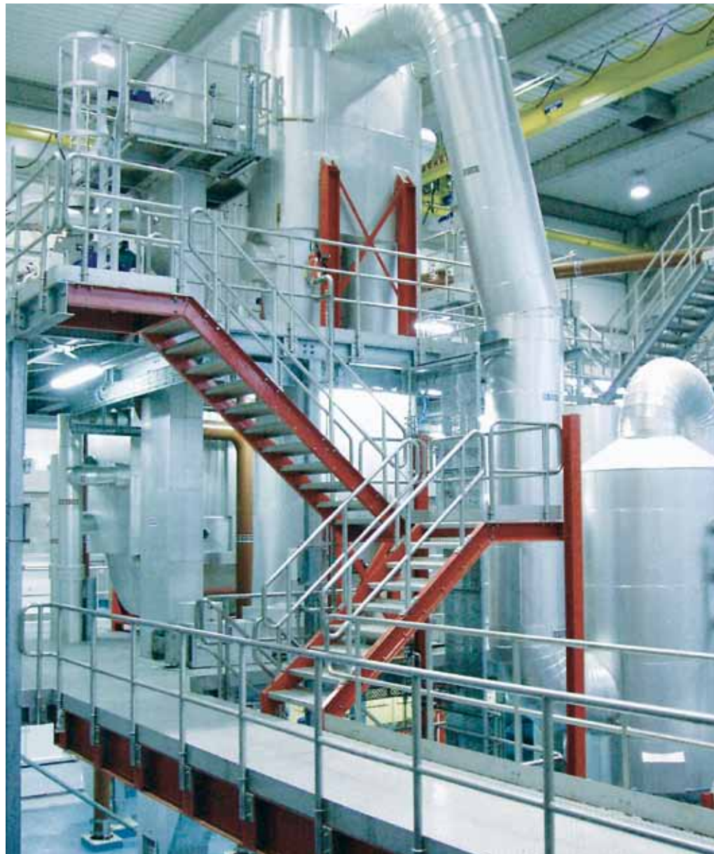
▲ Fluid bed dryer for sewage sludge in Leuven, Belgium.
