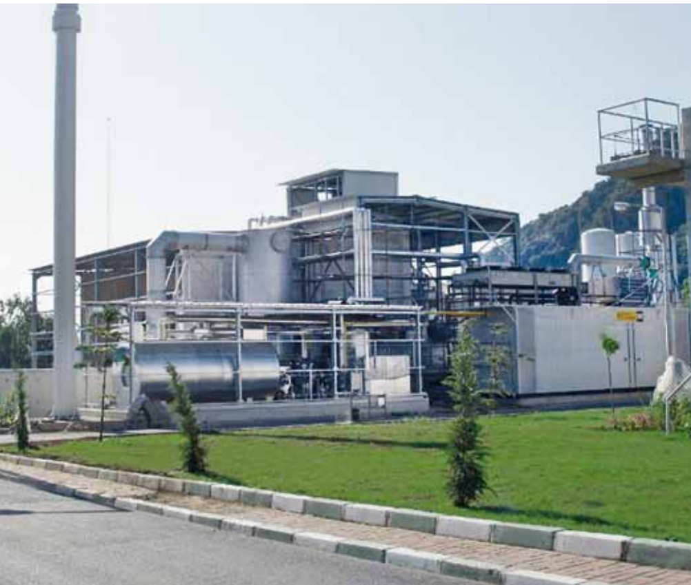
◀ Belt drying plant for sewage sludge in Antalya, Turkey
