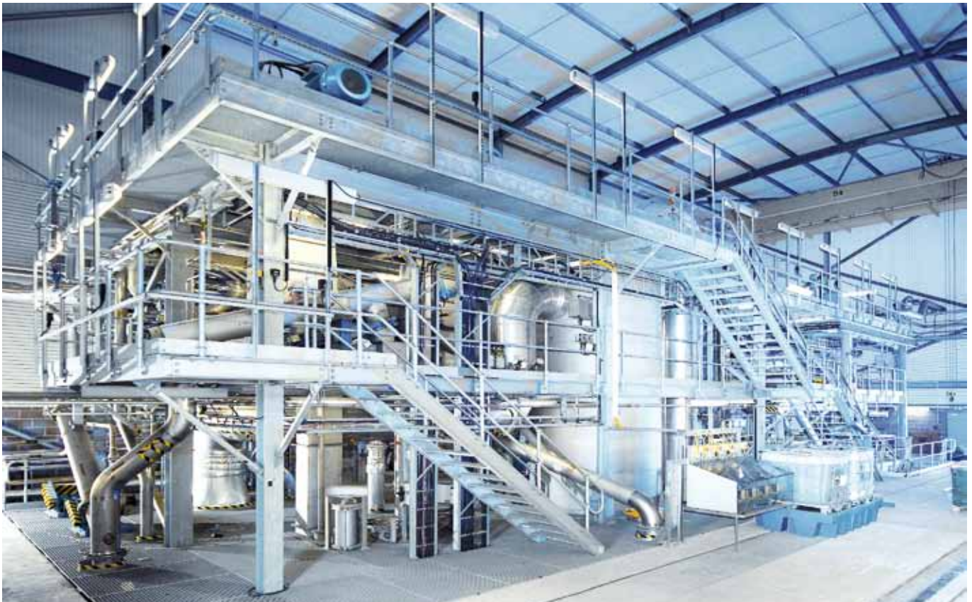
▲ Drum drying plant consisting of one line DDS 70 for drying of municipal sludge
