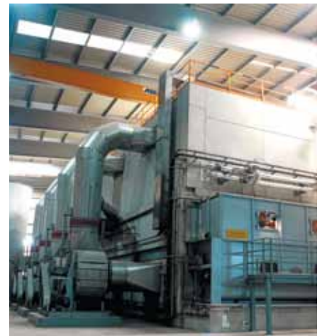
▲ Belt dryer in full concrete casing
