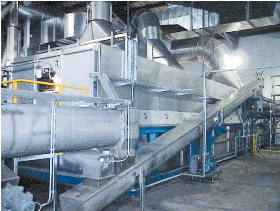
▲ Belt drying plant for fermentation residues in Leonberg, Germany
