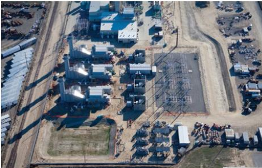
1. Turlock Irrigation District's Almond Plant added three fast-start LM6000PG peakers, but had to modify the SCR control logic for compatibility with 10-min start and remote dispatch
