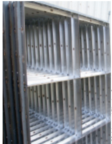
4. Framing for new static (barrier)-type filters is of stainless steel to minimize corrosion potential
