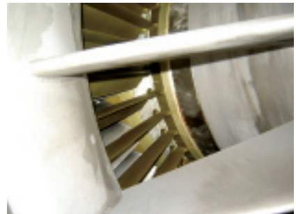
13. Unit 2 compressor inlet like new after 10,600 hours of operation with HEPA filters
