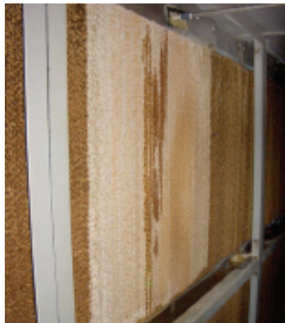
8. Microbiological fouling reduces efficiency and media life, can produce objectionable odors downstream, and can promote corrosion of framing
