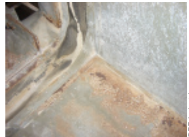
5. Corrosion of air-inlet floor must be addressed to prevent metal from flaking off and being ingested by the gas turbine
