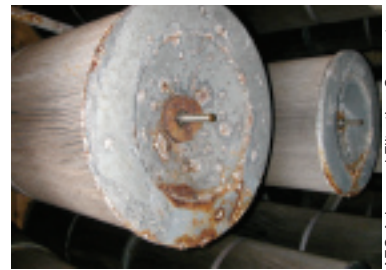
3. Galvanic corrosion from moisture ingress quickly chewed up metal portions of the original pulse-type filters
