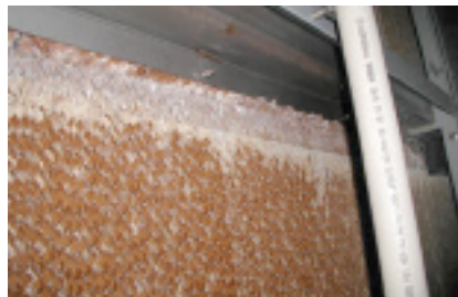
7. Scaling at the top of the media (frosty deposit) impedes proper operation of an evap cooler
