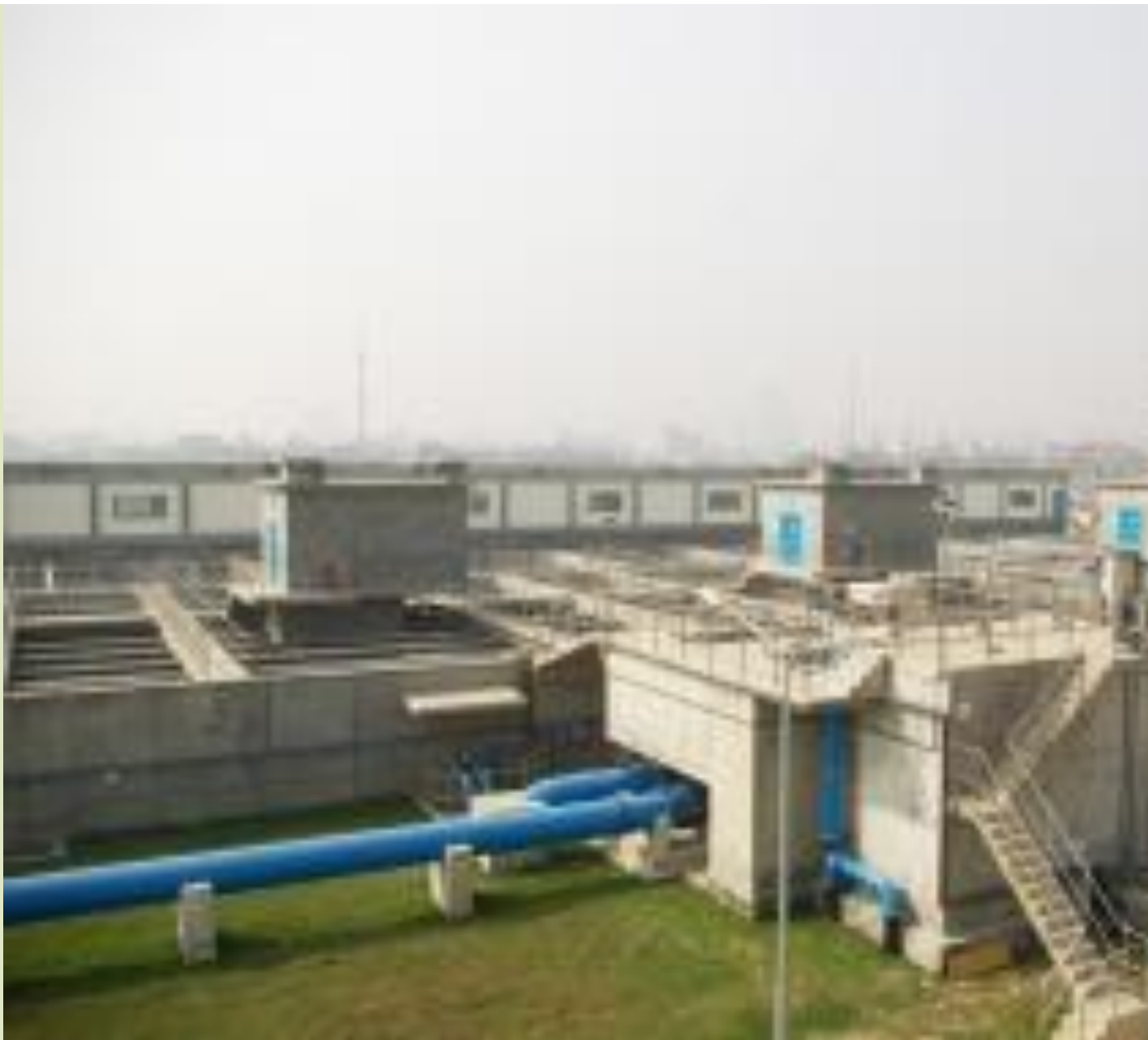
• case study Saidabad drinking water plant (Bangladesh)
