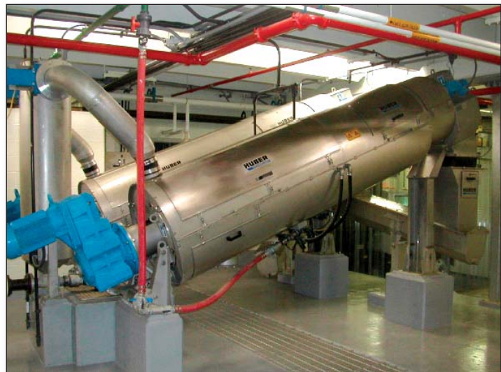
Installed incline screw press at Old Town Water Pollution Control Facility. (Atherton et al., 2005)
