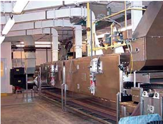
Burch BioWave ® dryer installed
