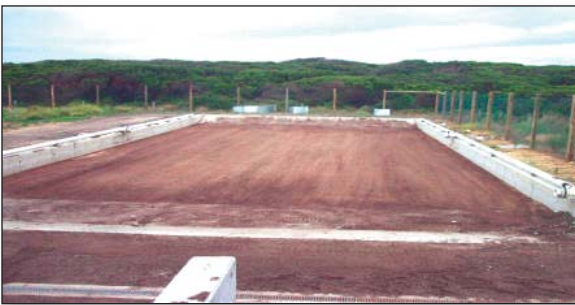
Deskins Quick Dry Filter Bed
