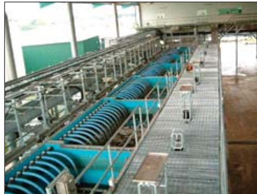
MBR Technology at Cauley Creek WRF Fulton County, GA
