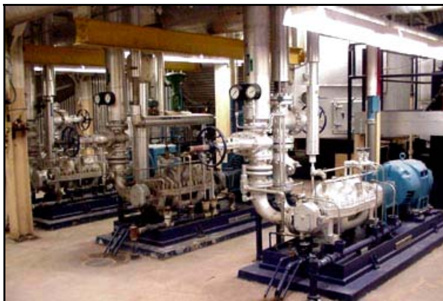
Figure 2 – Unit 7 Boiler Feed Pumps
