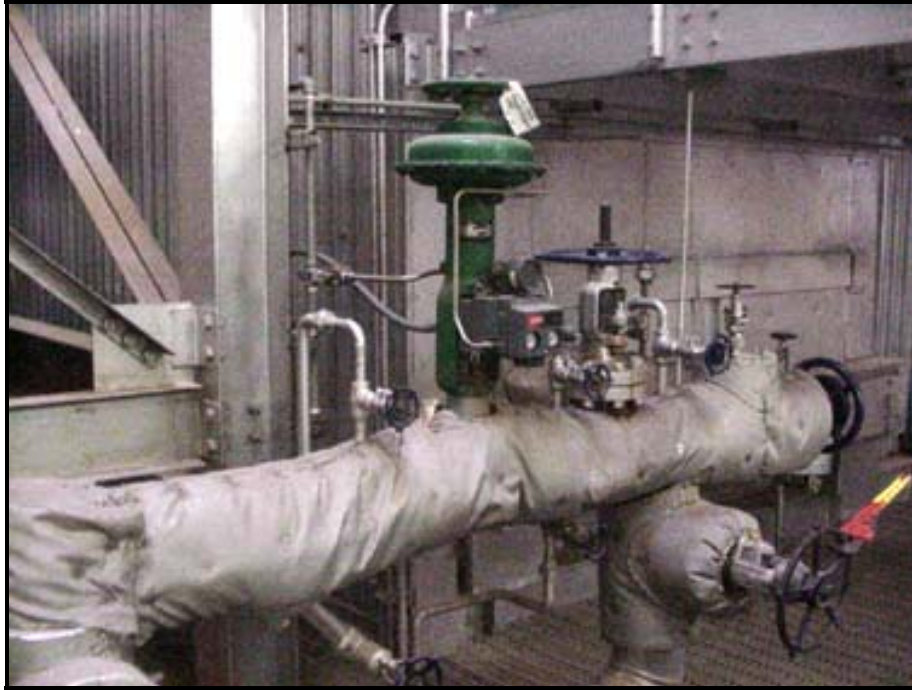
Figure 4 – Unit 6 Feedwater Control Valve
