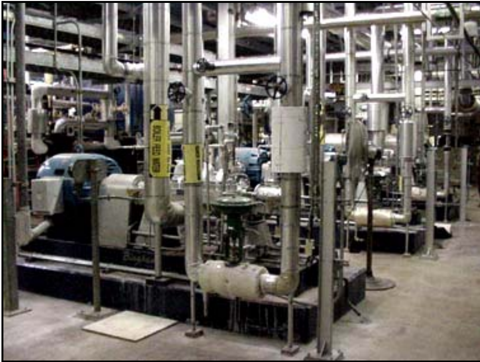
Figure 3 – Unit 8 Boiler Feed Pumps
