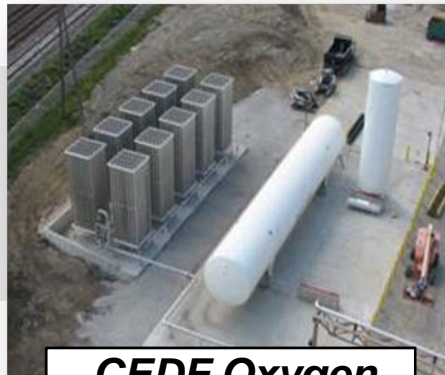
CEDF Oxygen Supply System
