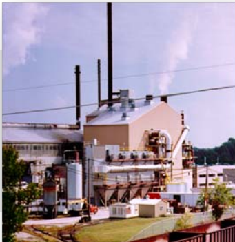
30 MWth Test Facility
