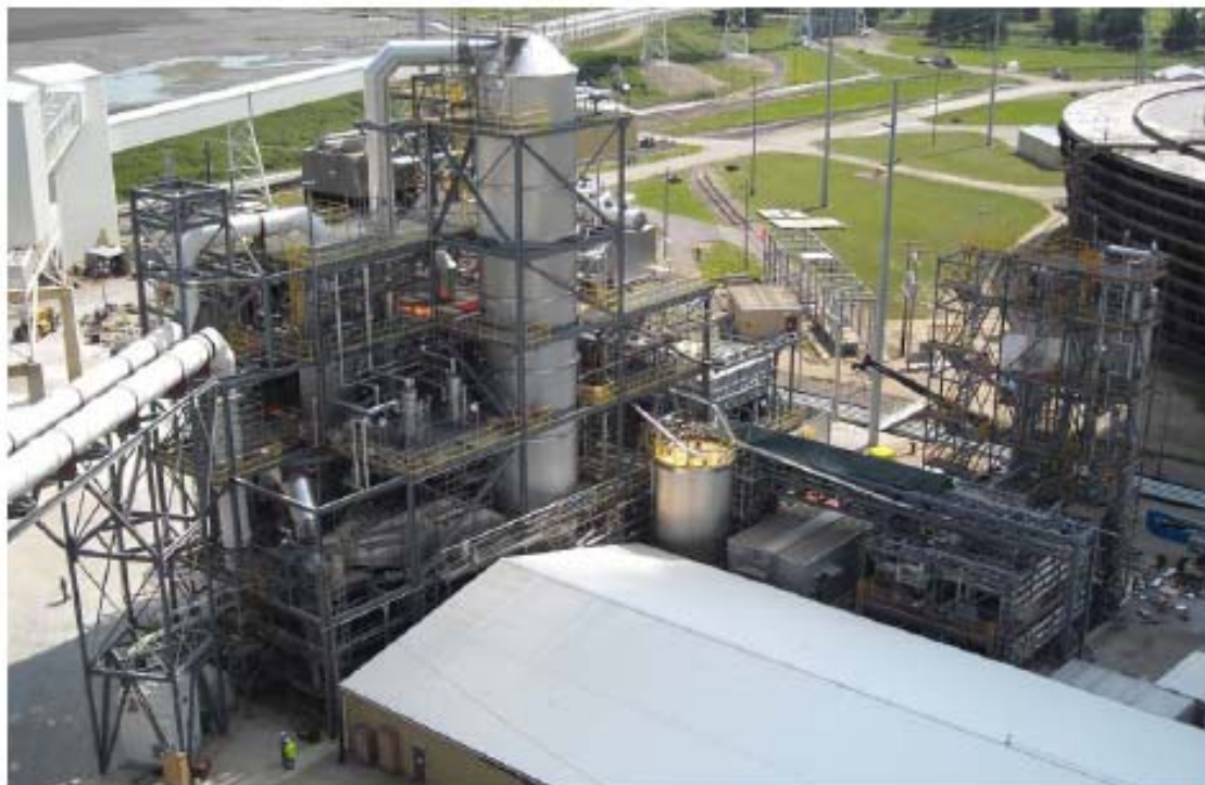
Alstom's Chilled Ammonia Process at AEP's Mountaineer Plant,
