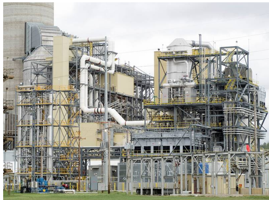
Alstom's Chilled Ammonia Process at AEP's Mountaineer Plant,
