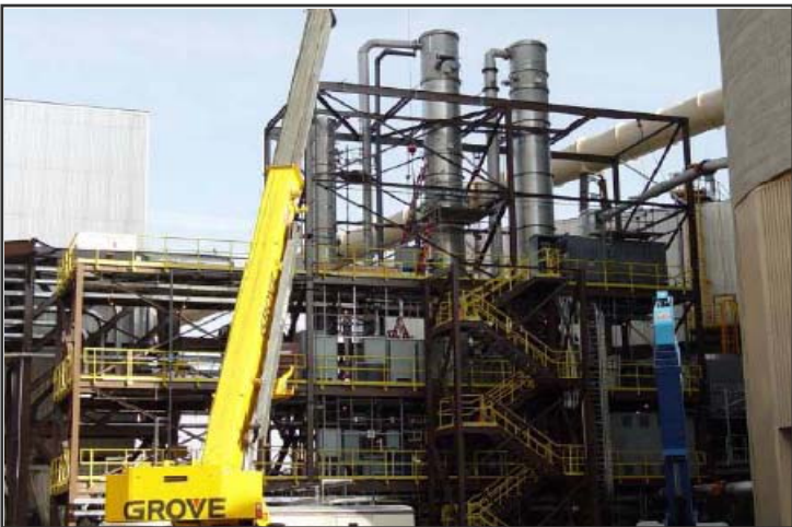
Test Bench 5 MW, start up in February 2008
