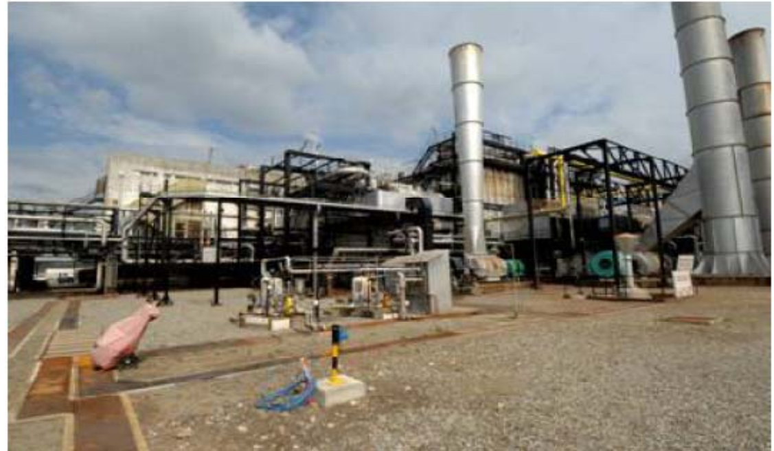
30 MWt demonstration – Lacq, France
